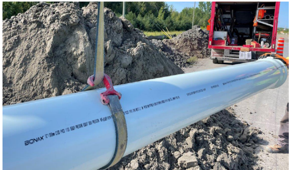
Testing 1km section of the pipe for a perfect seal before the next section.
