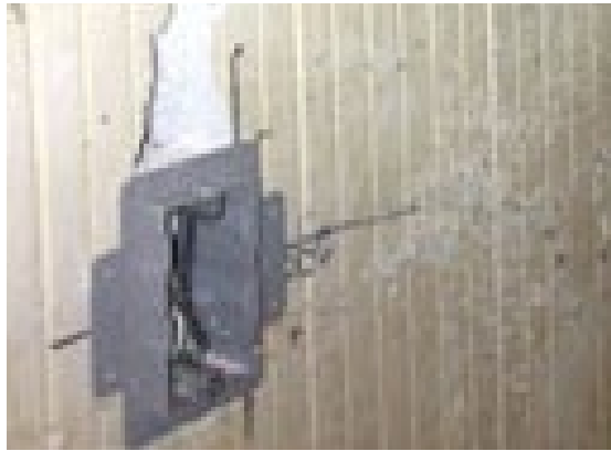
More than 700 electrical boxes were needed throughout the new hotel for power and data connections
