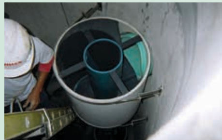
Stainless steel straps and epoxy painted walls for additional layer of corrosion protection, Charlotte, NC.
