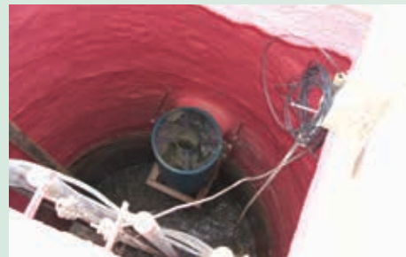
Vortex Flow operating in a pumping station wet well, Jacksonville, Florida.
