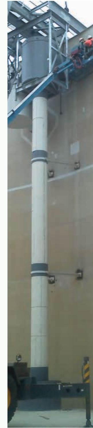
Vortex installed in 5 million gallon CSO storage tank adjacent to WWTP – Port Angeles, WA
